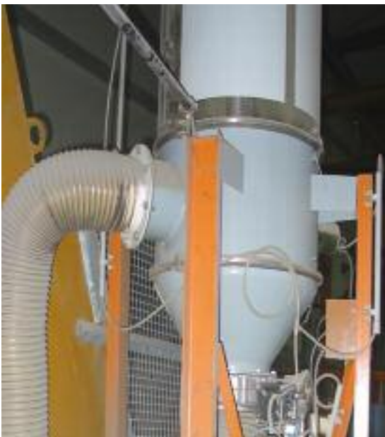
▲ Dust filter with reverse air shock filter cleaning
