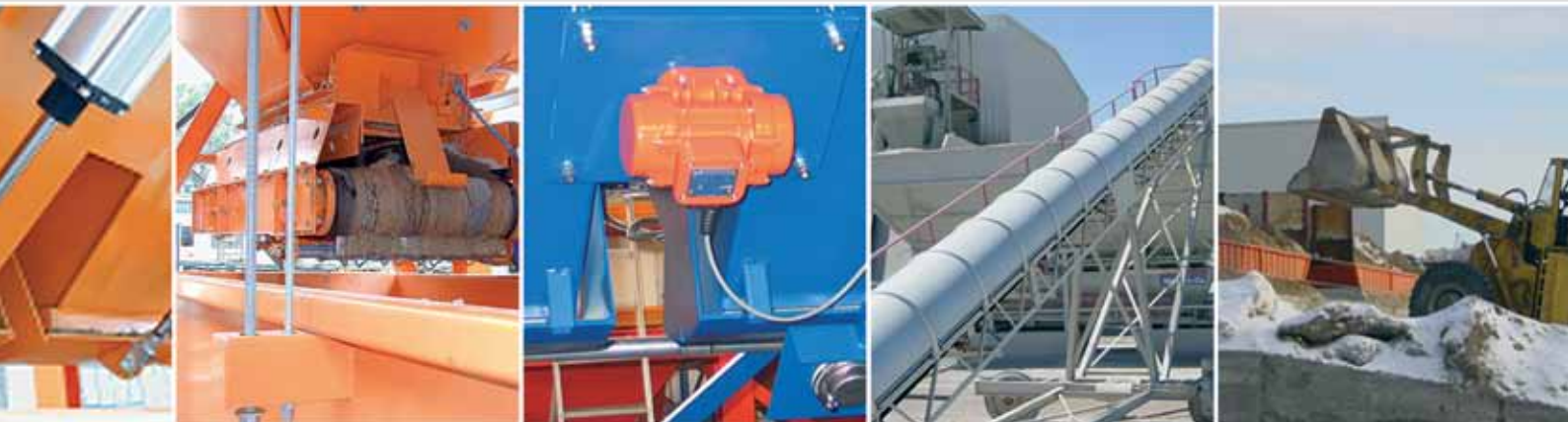
from row-type silo: batching gates for coarse / fine dosing, dosing belts, weighing platform and moisture measuring probe "Hydrotester"
