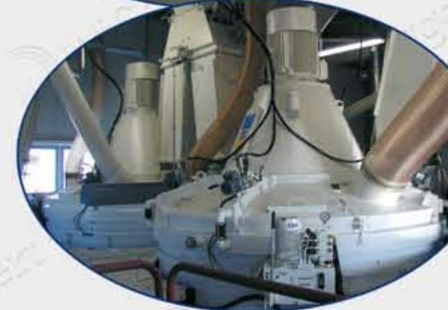
Large access doors for cleaning and maintenance
