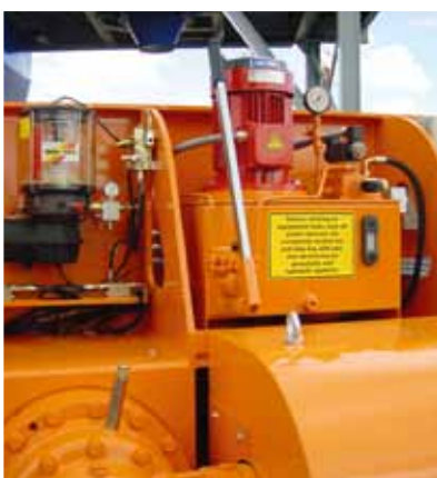
Hydraulic unit for actuation of the discharge gate
