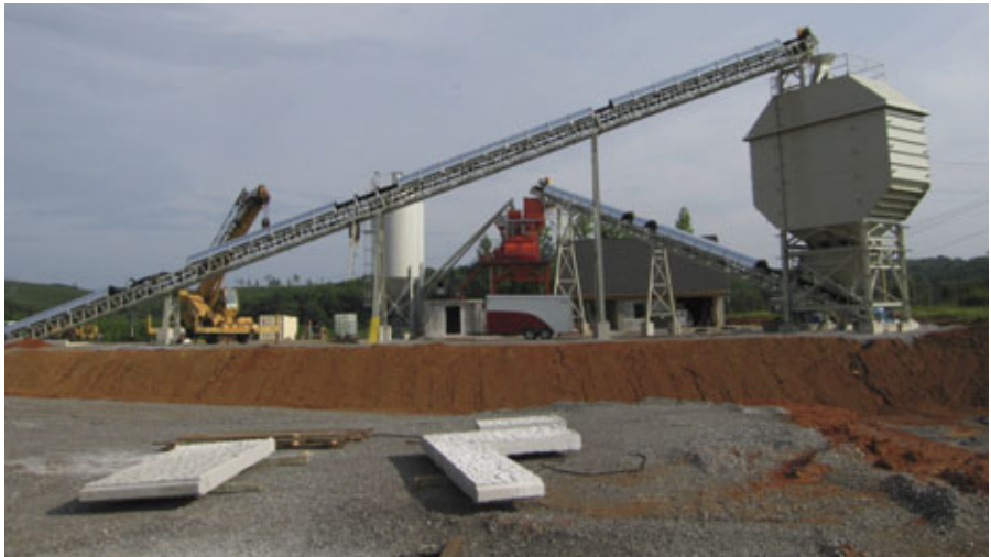
The new VanHooseCo combination ready-mix and precast tilt-up wall operation on 33-acre site in Loudon, TN. At right, 300-ton 5-compartment aggregate storage and in the back are cement silos and orange twin-shaft mixer platform.
