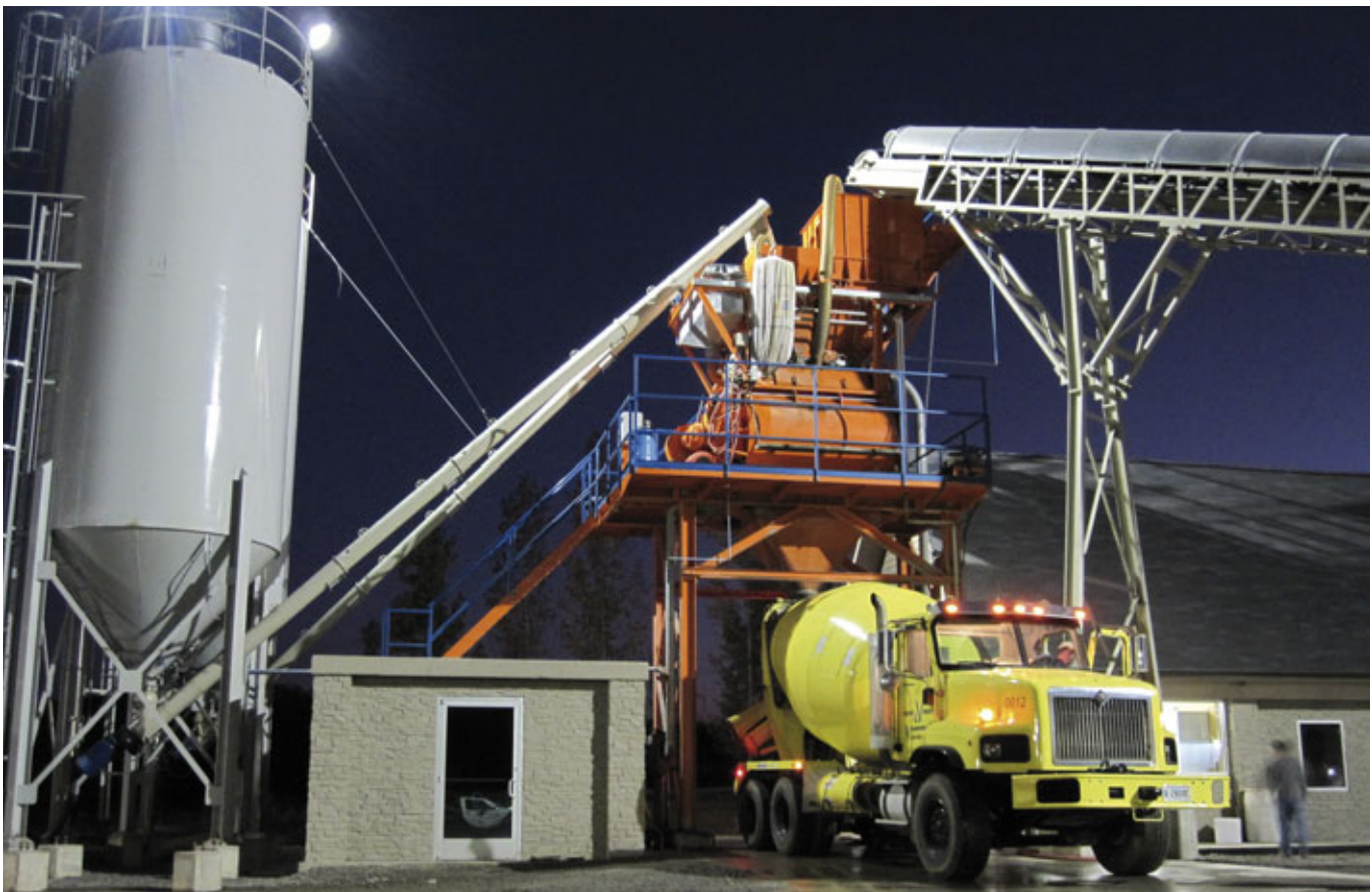
Like night and day – Centrally mixed RMC produced in VanHooseCo’s new ACT MobilMat batching plant provides superior consistency over dry batched RMC.
