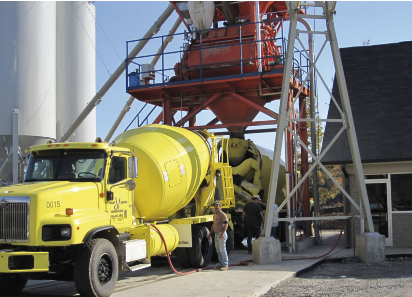
Two trucks queue up to be loaded from the ACT MobilMat Mo120 batch plant at VanHooseCo's RMC and precast tilt-up wall operation in Loudon, TN.
