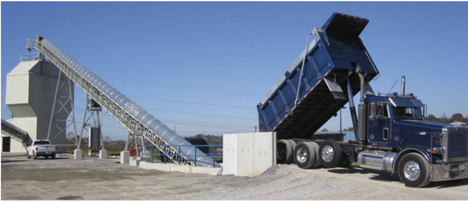
In-ground truck dump hopper allows aggregate deliveries to be transferred via 300 ton-per-hour conveyor from ground level to the aggregate storage bins (at left) without a front-end loader – a 5-way turn head directs different aggregates into appropriate storage bins.
