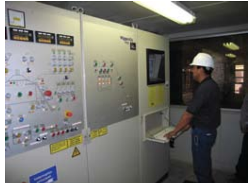
PCS Windows-based Control
