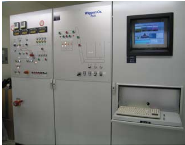
PCS Windows-based Control
